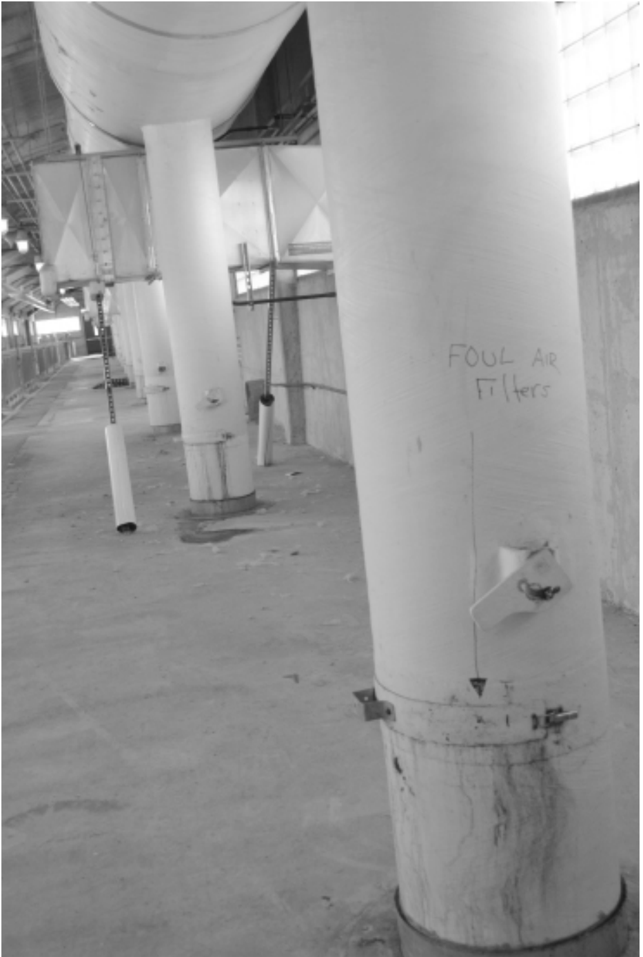
Wastewater treatment plant, photo by Johanna Oppeck
